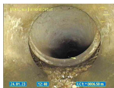
Pipe requiring renewal works
